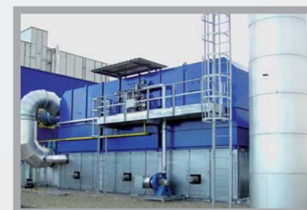
RTO for V.O.C. exhaust from alucans lining
