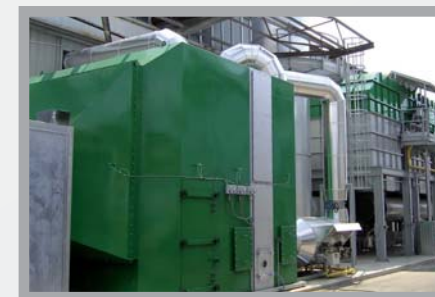
Concentration Unit for V.O.C. coming from plastic components painting
