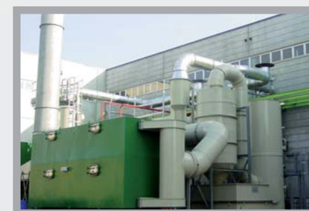
Scrubbers for inorganic wet absorption and final stage of V.O.C. cleaning by using activated carbon
